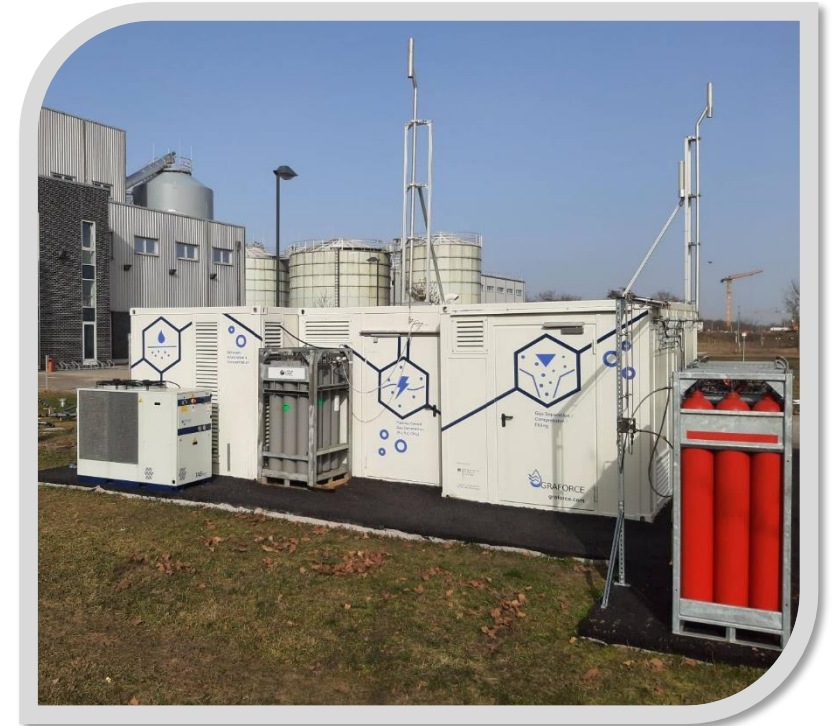
Graforce hydrogen plant from ammonia feedstock
