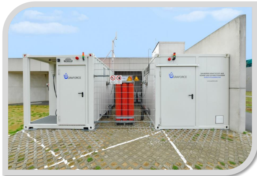
Hydrogen fuel plant from natural gas feedstock
