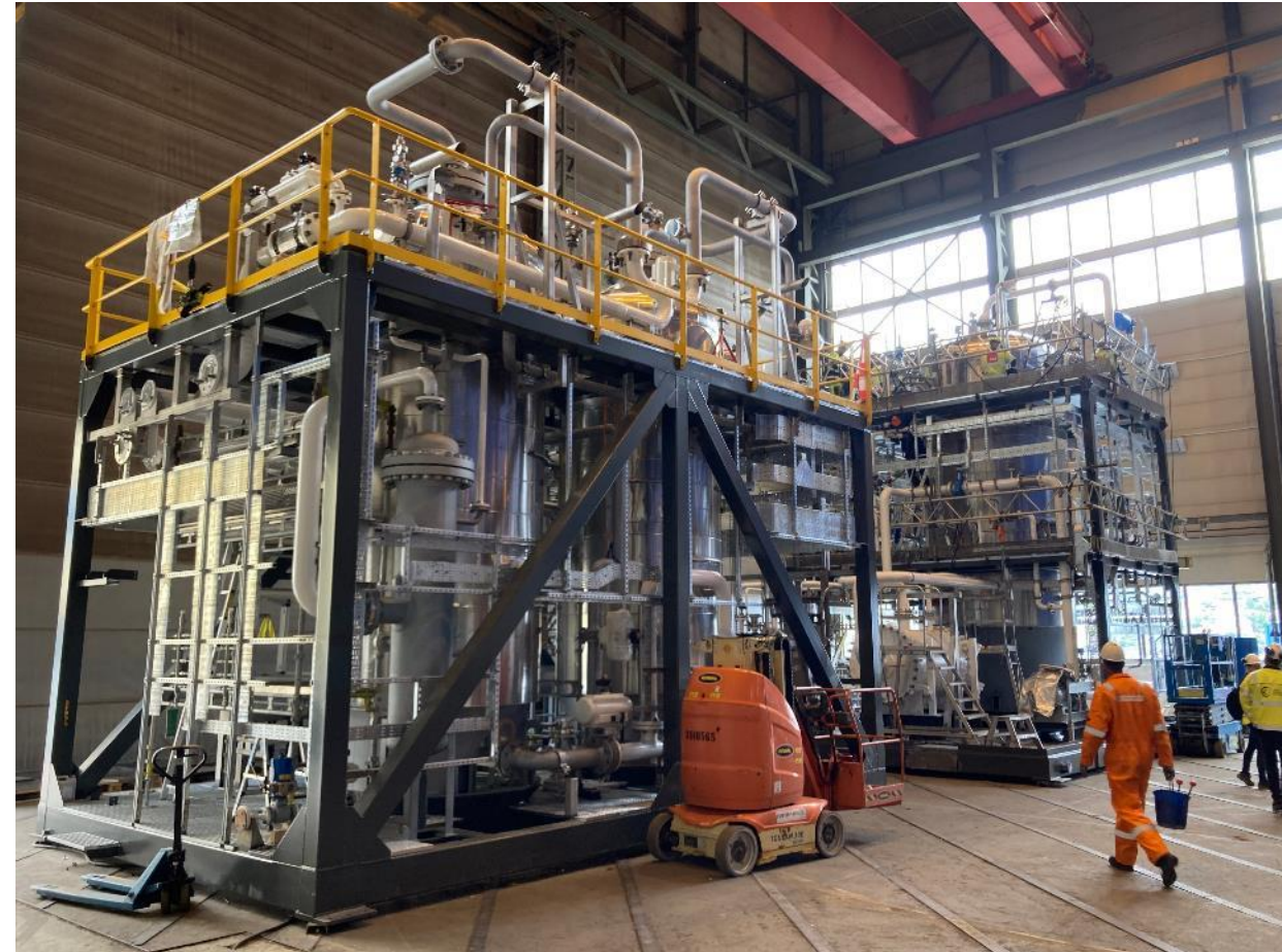
Drying and reclaimer package
