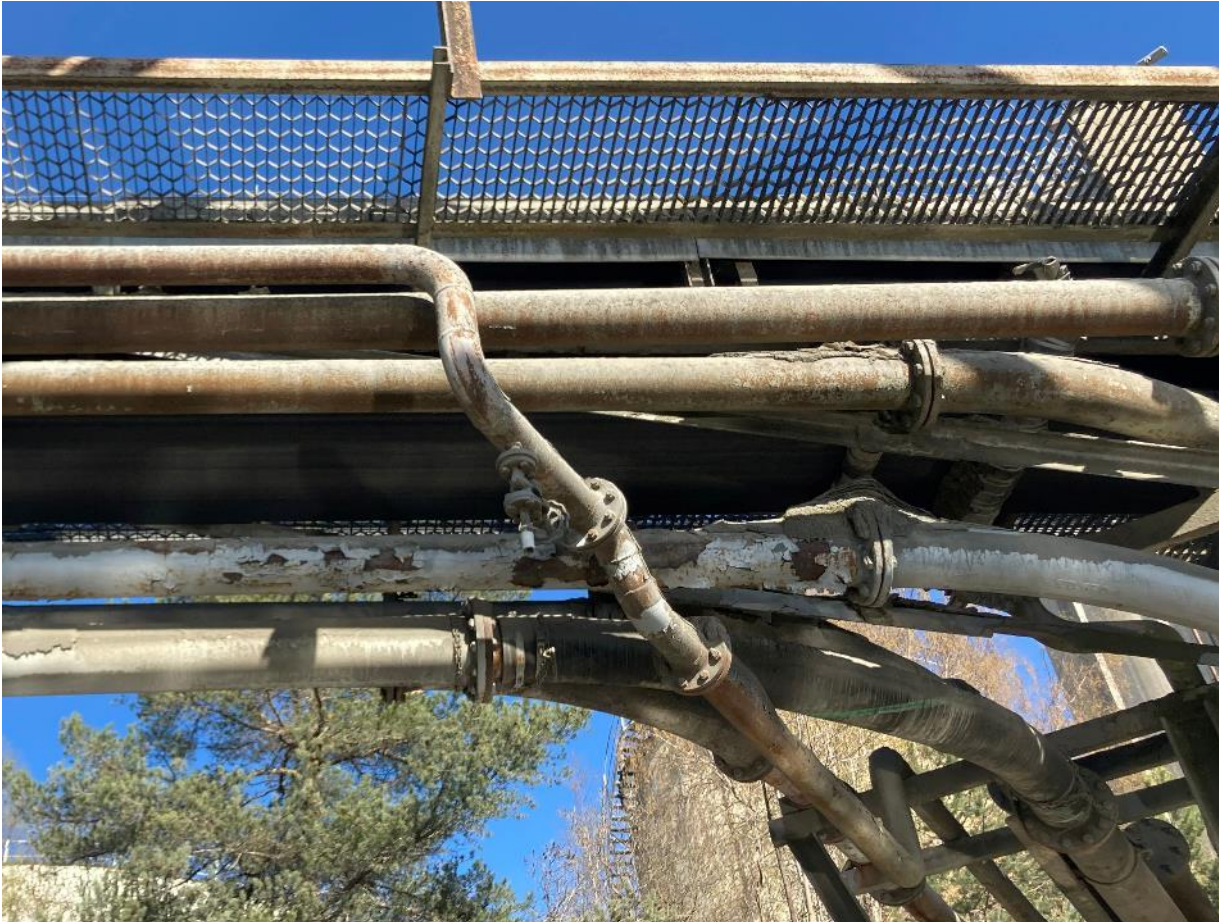
Carbon steel, crude supports etc (cost-effective focus)
